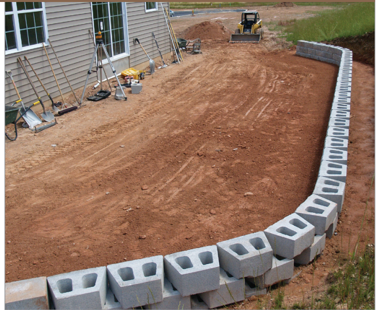
The house featuring the Anchorplex™ retaining wall system sold quickly because potential buyers saw an expanded, flat usable backyard.
